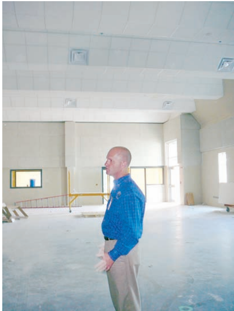
Shane Jones, LISD business manager, explains about the special ceiling to help with the acoustics in the band hall.
