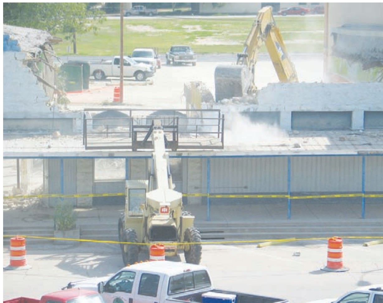
The historic Brooks Supermarket building on Courtyard Square was demolished to make way for an addition to the new Lamparasas County Office Building.
