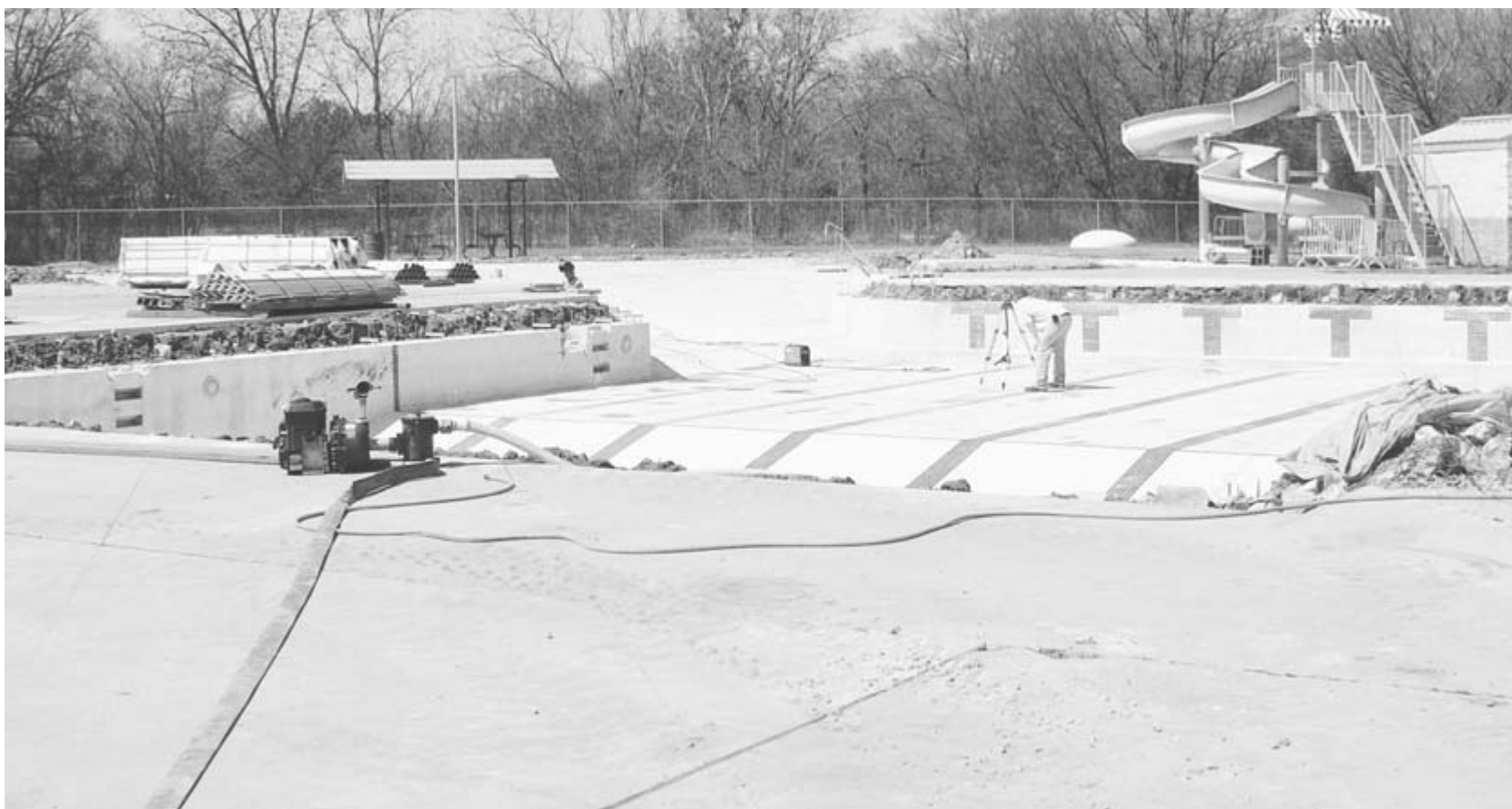
Repairs to the Hanna Springs Swimming Pool were ongoing throughout last year.
